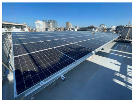
T's eco Kawasaki Solar Panels
