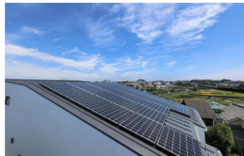
Solar power generation system
