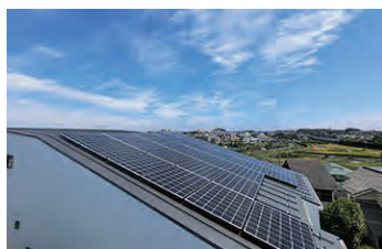
Solar power generation system
