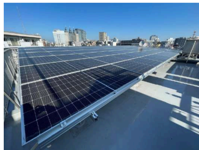
T's eco Kawasaki solar panels
