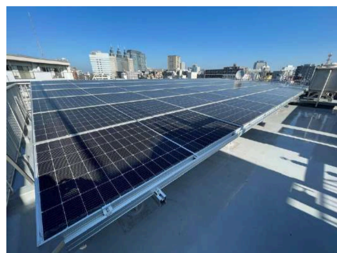
Solar panels installed on the rooftop
