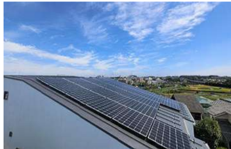
Solar power generation system
