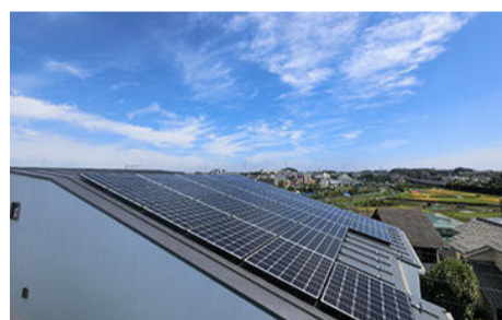
Solar power generation system
