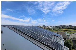
Solar power generation system
